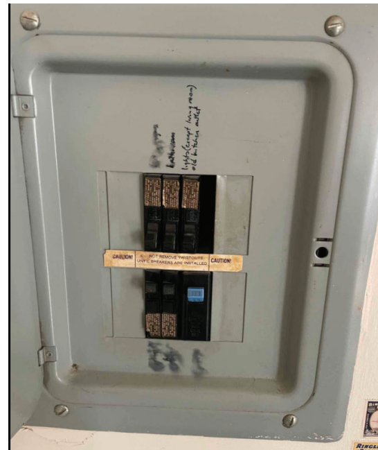
Insufficient Amperage Little Expansion Space
