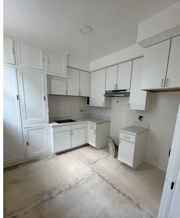
Upper Units Kitchen
