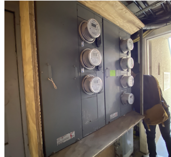
Insufficient Clearance Encroaching on Egress
