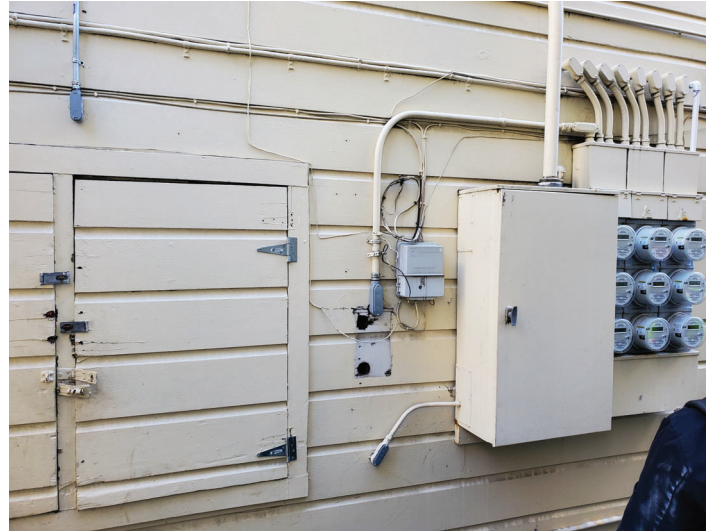
Outdoor With Sufficient Service Clearance
