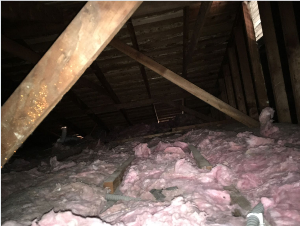
Today: Attic, R-19 insulation Recommend: R-38
