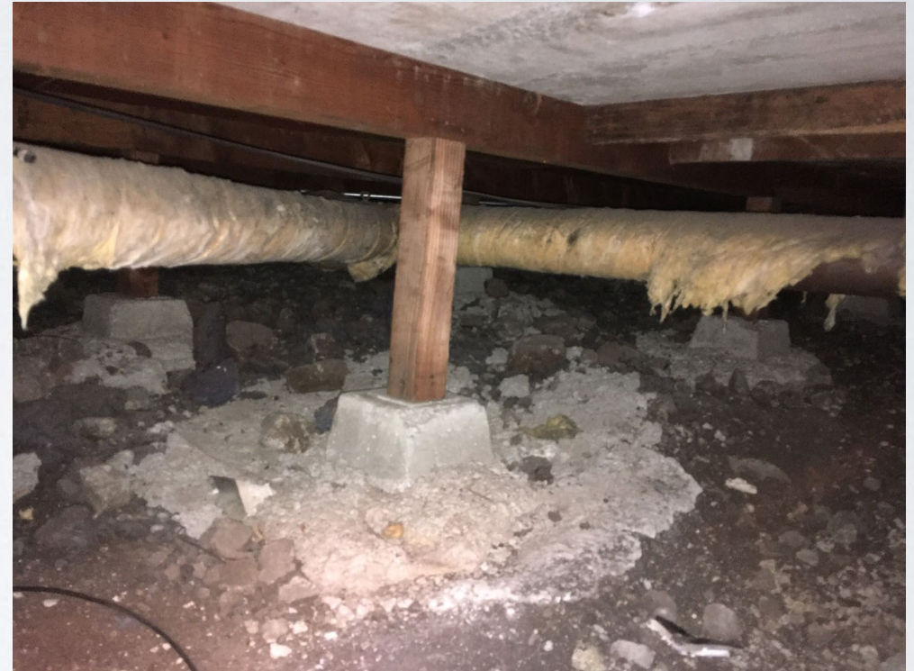
Today: Crawlspace, no insulation, poorly insulated ducts Recommend: R-19 or R-30 for floors, repair ducts
