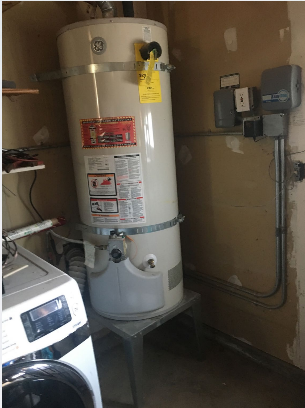
Today: 50-gallon gas tank WH in garage
